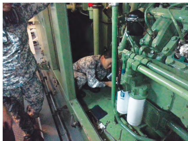
Figure 1. An RSN Marine Engineer working on a DG
